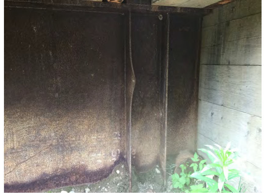
Damage noted to left downstream stiffener
