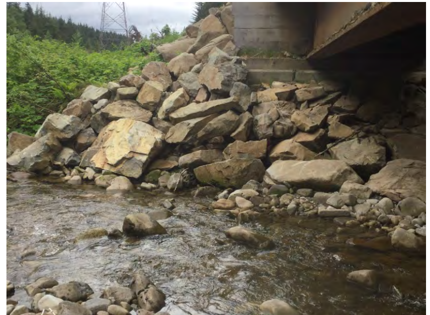
Slight riprap scour right downstream bank
